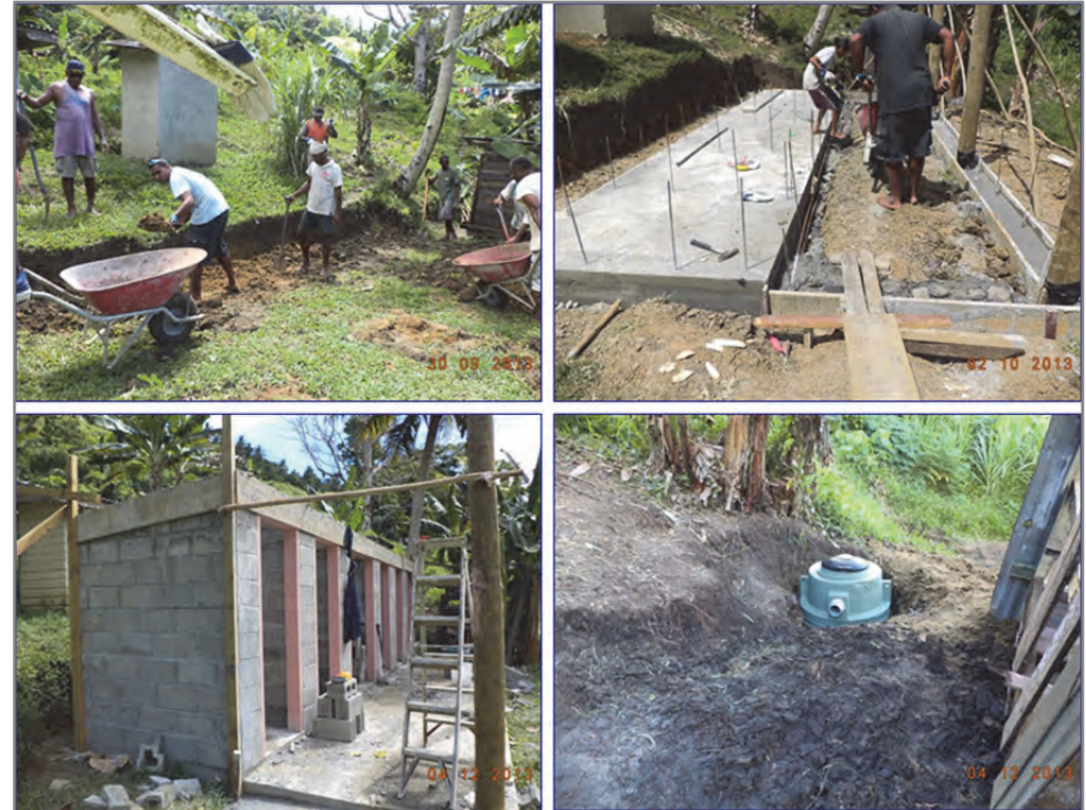
Local villagers helped to dig the foundations, sewerage system and the water pipe trenches
